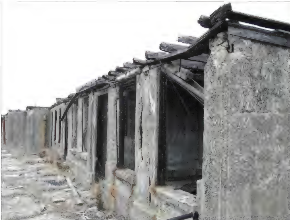
Figure 5.62. Plotting rooms, Battery Potter. In improving physical access to the upper level of Battery Potter for use as an elevated prospect, rehabilitating the deteriorated plotting rooms shown here may be of some value for interpretive purposes. Once the roofs of these buildings are replaced, the interiors may be used to house durable exhibitry. Enamelled interpretive wayside panels may effectively substitute for missing window frames, offering detailed graphic interpretation of Battery Potter and the entire coastal defense system (Olmsted Center, January 2009).
